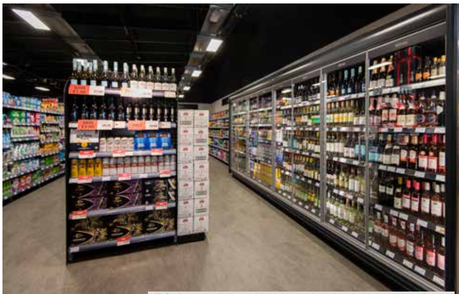
"F Gas" energy efficient refrigeration has been installed in a number of stores.
